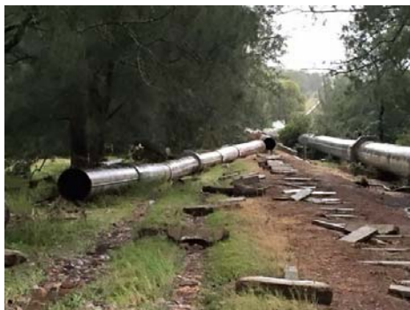
Section of HWC CTGM Washed away during the storm
